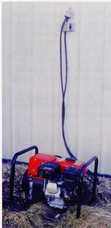
Back-up power for ventilation fans in wintering room.
