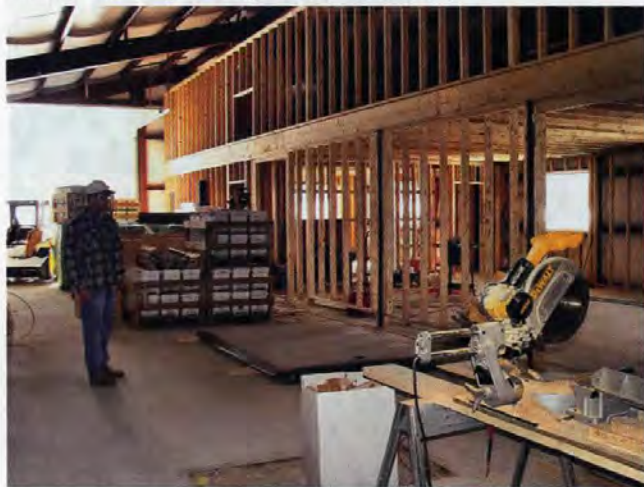
A new Swan's Honey packing facility is under construction in Albion, Maine. (photo by Karen Baldauski)
