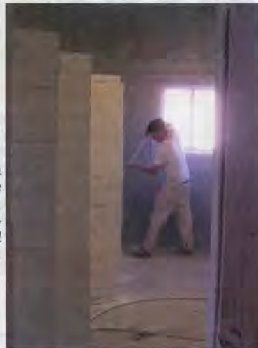
The Paint room is located in the workshop building, where equipment is assembled, trucks repaired, boxes preserved, the crew meets, and some equipment is stored.
