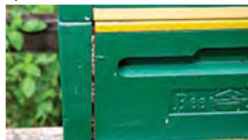
Figure 4. A cracked joint. My fault. I should have applied glue at the time of assembly.
